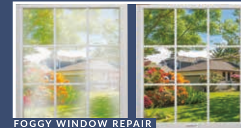
FOGGY WINDOW REPAIR
